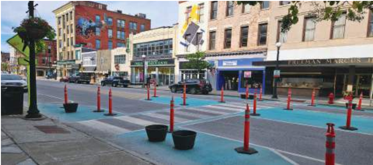
A direct action using paint and plastic bollards, facilitated by Brian Budrow, DRP, RRPC, and DPW ©CORI
